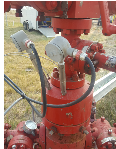
Figure 1.3: The cable connections from two down-hole gauges coming out of the Christmas tree.
